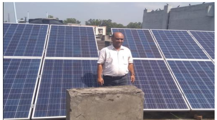
Fig(3) (Installed solar panel)
